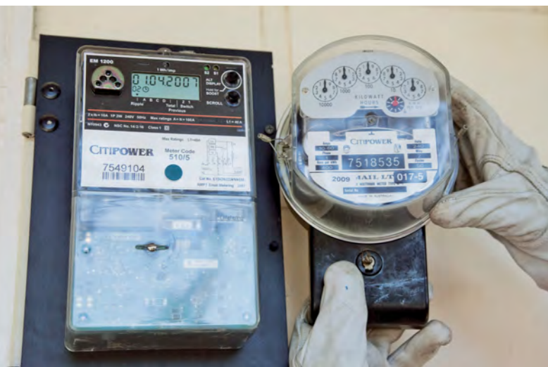
THE OLD METERS WERE READ FOUR TIMES A YEAR. THE NEW ONES TRANSMIT CONSUMPTION DATA EVERY 30 MINUTES TO THE ENERGY SUPPLIER'S CONTROL CENTER.
